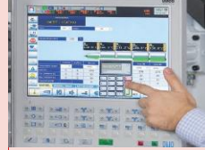
TOUCH SCREEN CONTROL PANEL. DOKUNMATİK KONTROL PANELİ.
